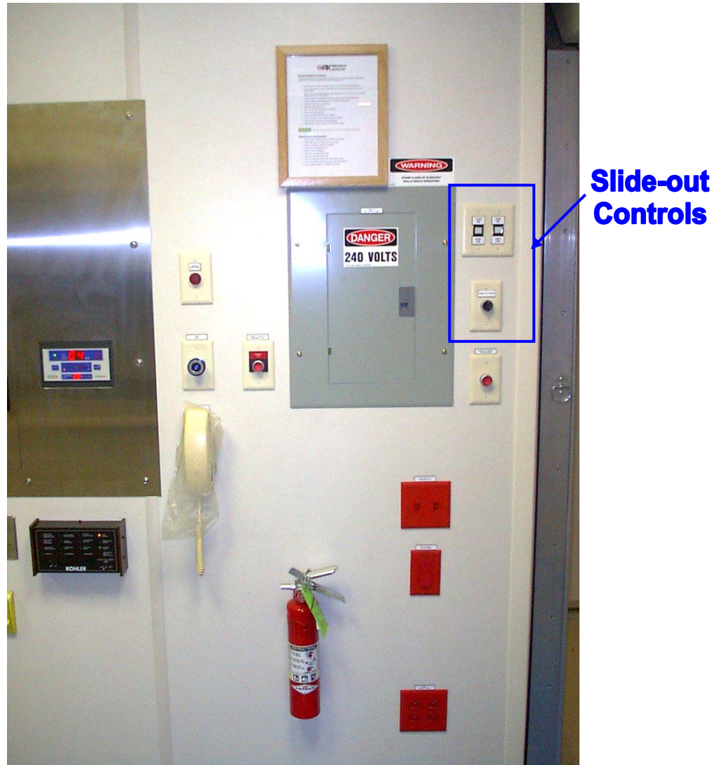
Figure 11: Procedure Room Controls
