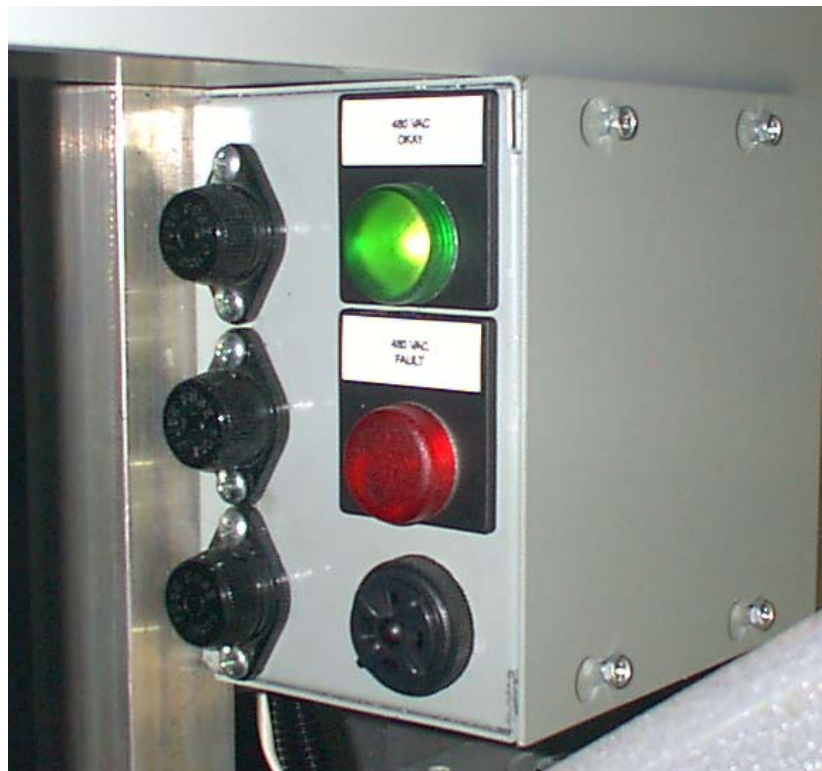
Figure 48: 480V AC Phase Power Monitor
