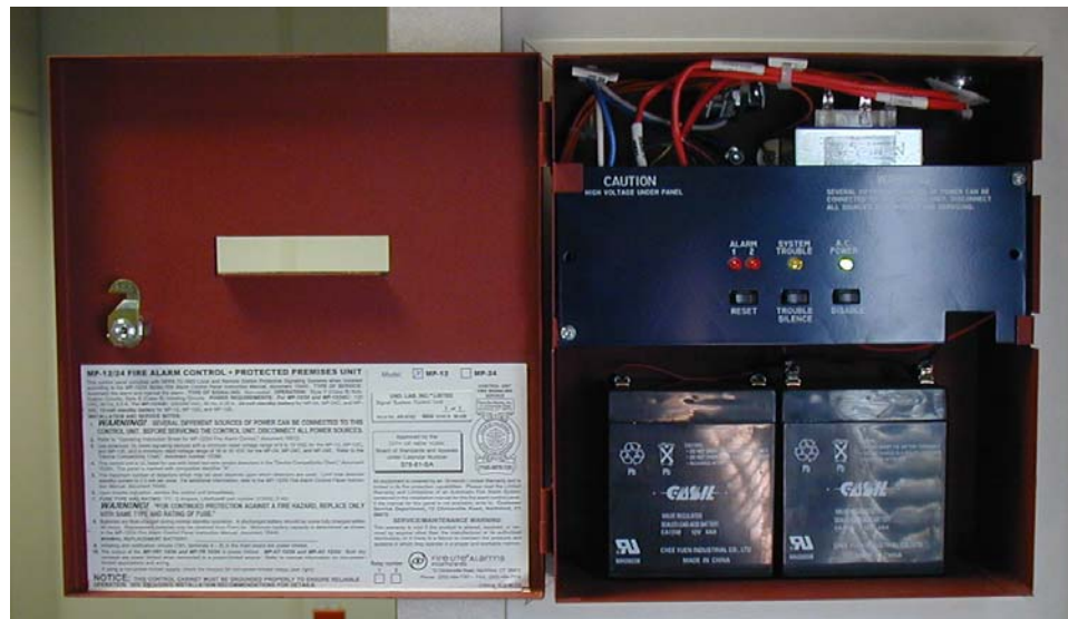
Figure 3: Fire Alarm Control Panel
