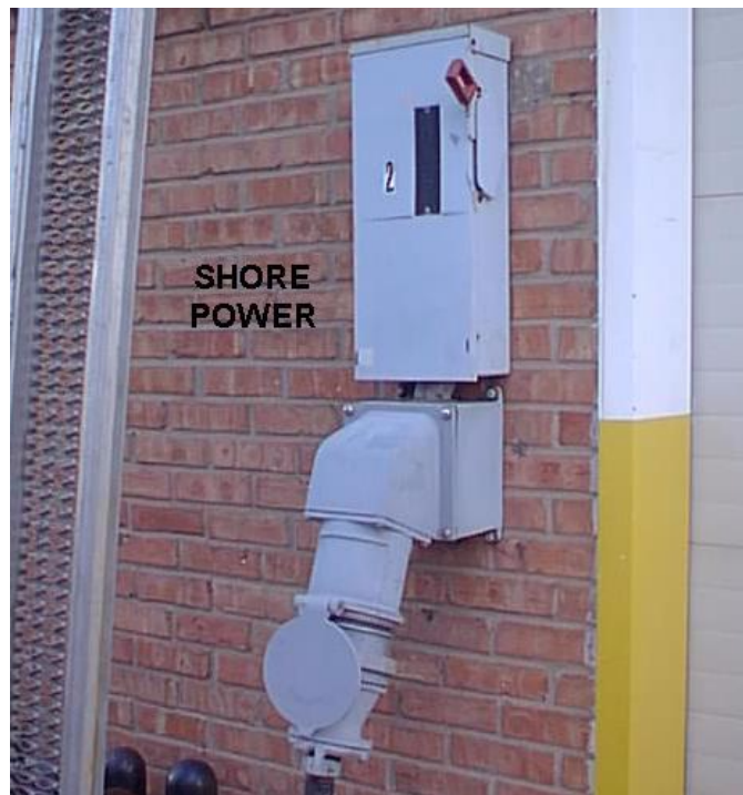
Figure 8: Shore Power Connection.
