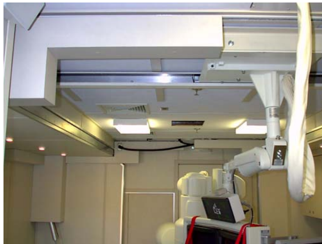
Figure 64: Procedure Room Lighting
