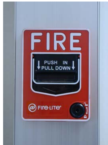
Figure 33: Fire Alarm Pull Station
