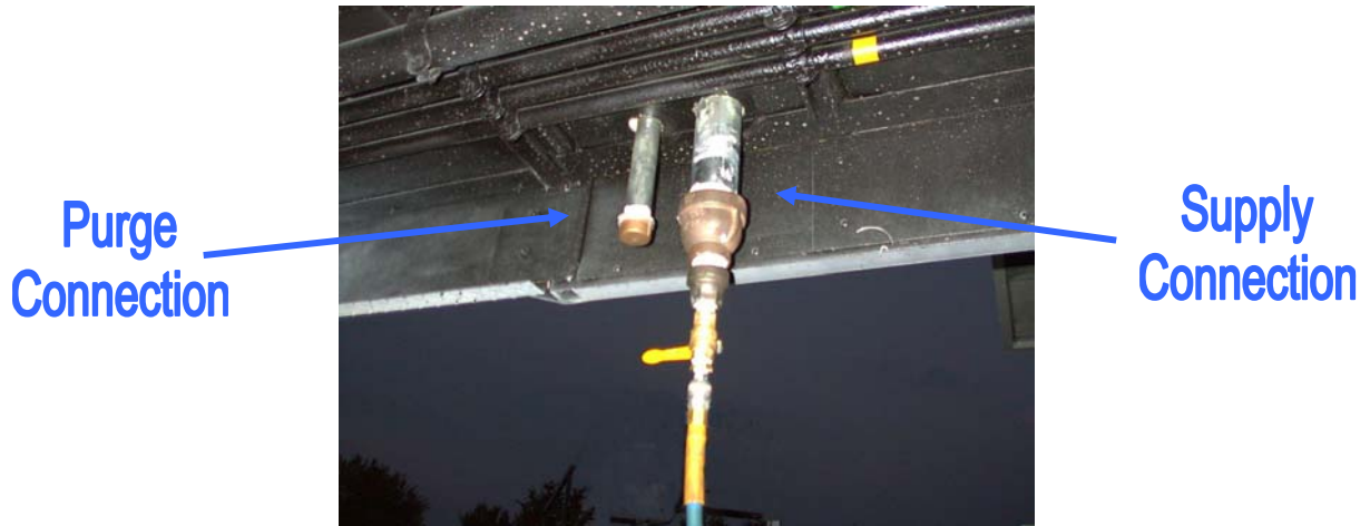
Figure 38: Fire Suppression Supply and purge connections
