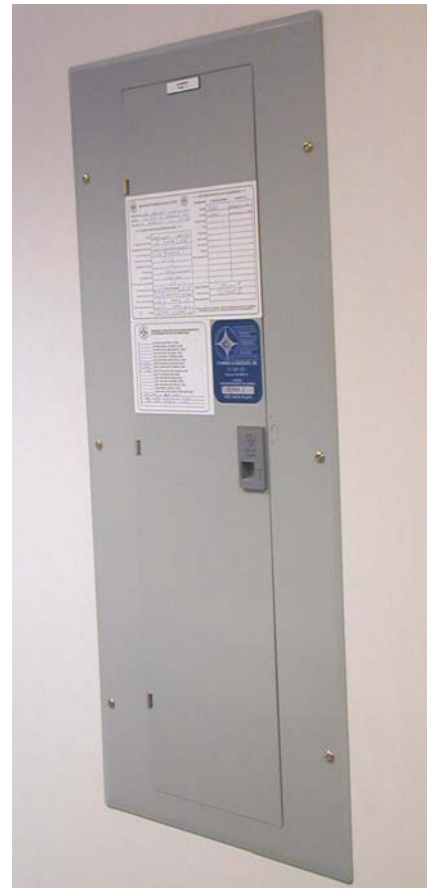
Control Room Panel
