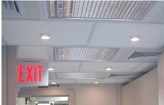
Figure 63: Control Room Lighting
