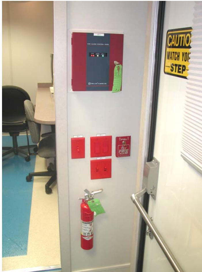
Figure 10: Control Room Controls
