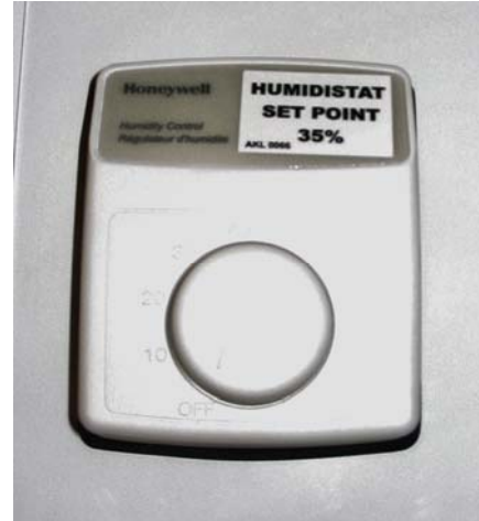
Figure 28: Humidistat Temperature Control
