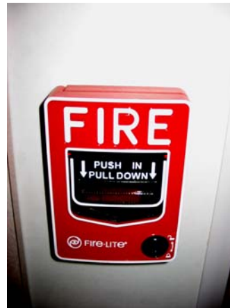
Figure 19: Fire Alarm Pull Station
