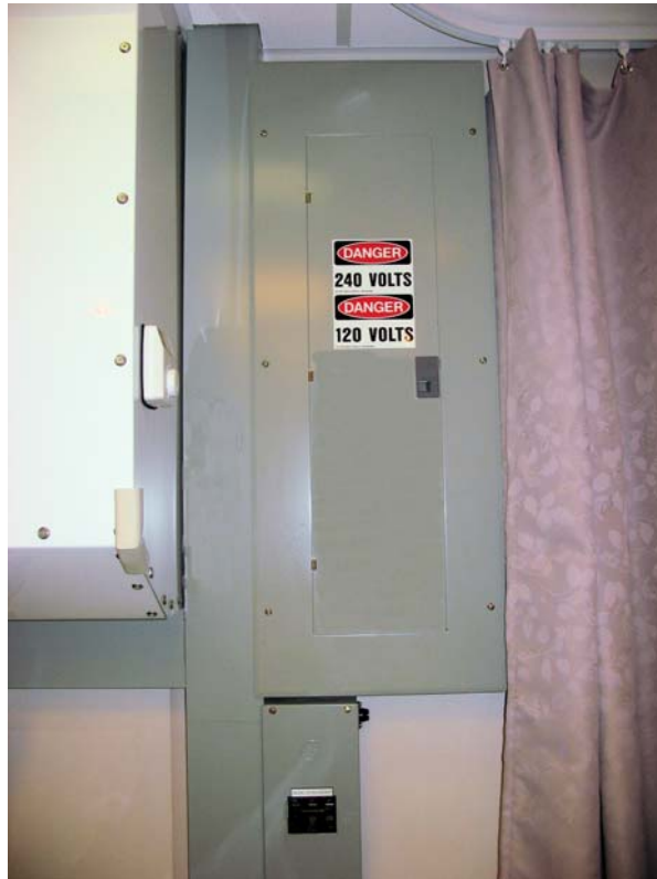
Figure 22: 120/240V AC Electrical Panel
