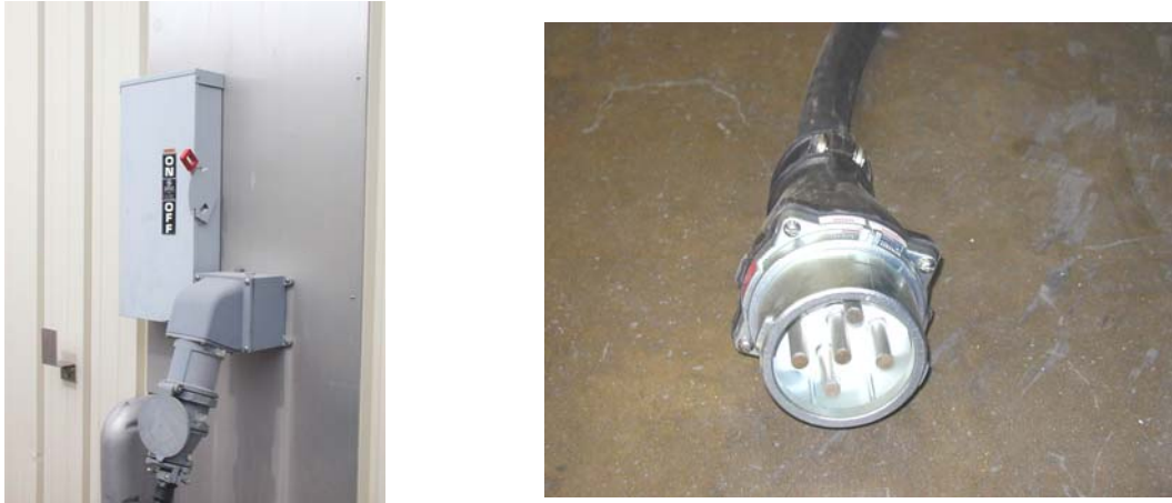
Figure 23: Shore Power Connection
