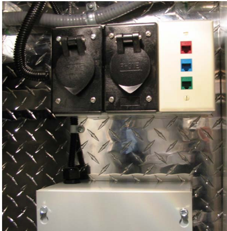
Figure 9: Phone & Data Line Connections
