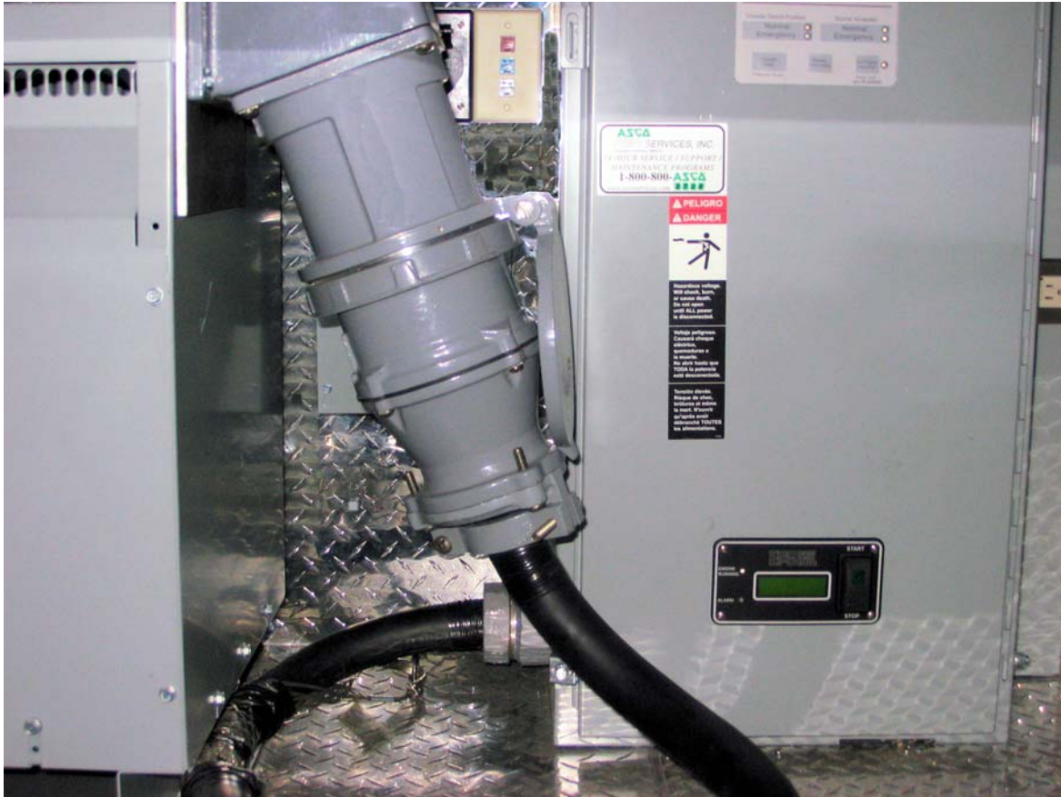
Figure 21: 240V AC Electrical Panel Automatic Transfer Switch
