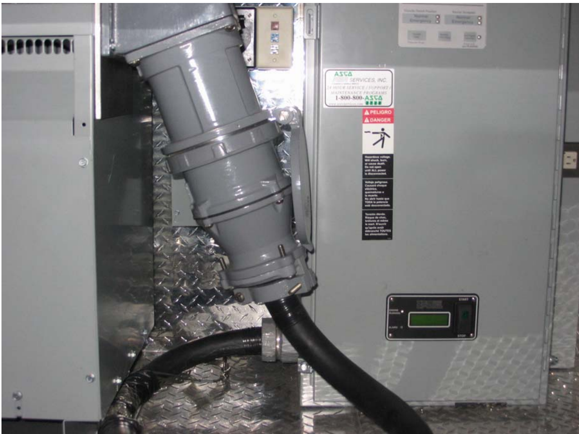
Figure 25: Automatic Transfer Switch (ATS)
