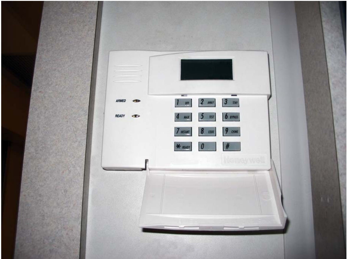
Figure 30: Intrusion Alarm Keypad
