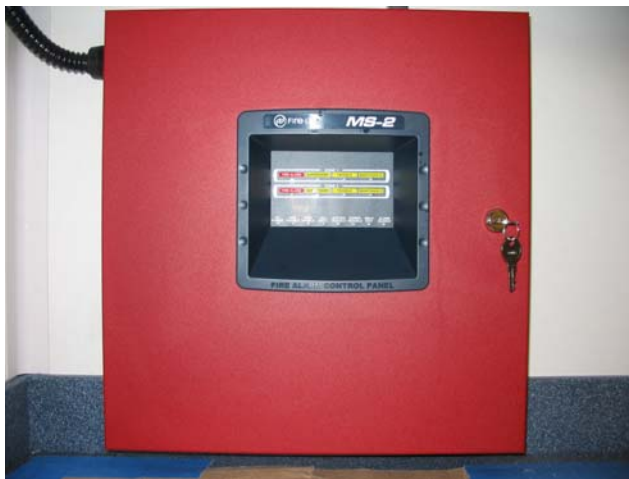
Figure 18: Fire Alarm Control Panel
