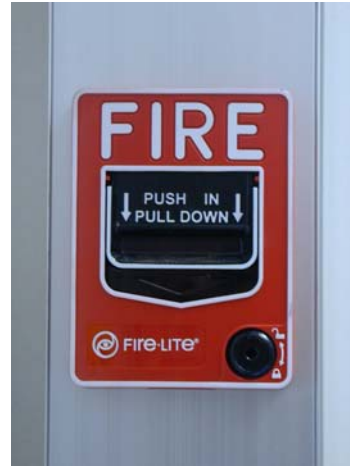
Figure 20: Fire Alarm Pull Station
