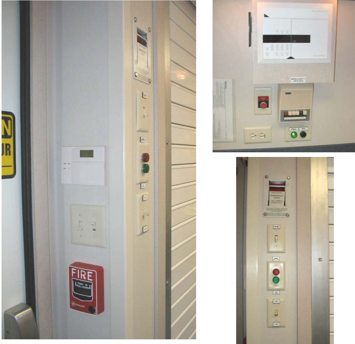
Figure 11 Mobile Unit Controls
