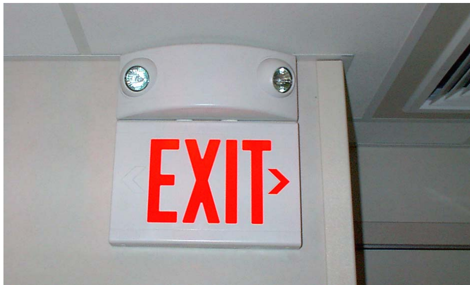
Figure 16: Control Room Emergency Lighting
