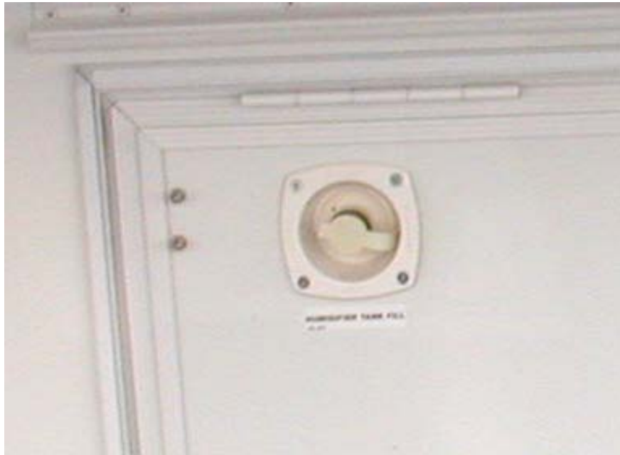
Figure 26: Humidifier Tank Fill
