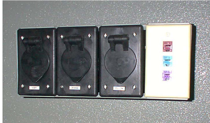
Figure 12: Phone & Data Line Connections
