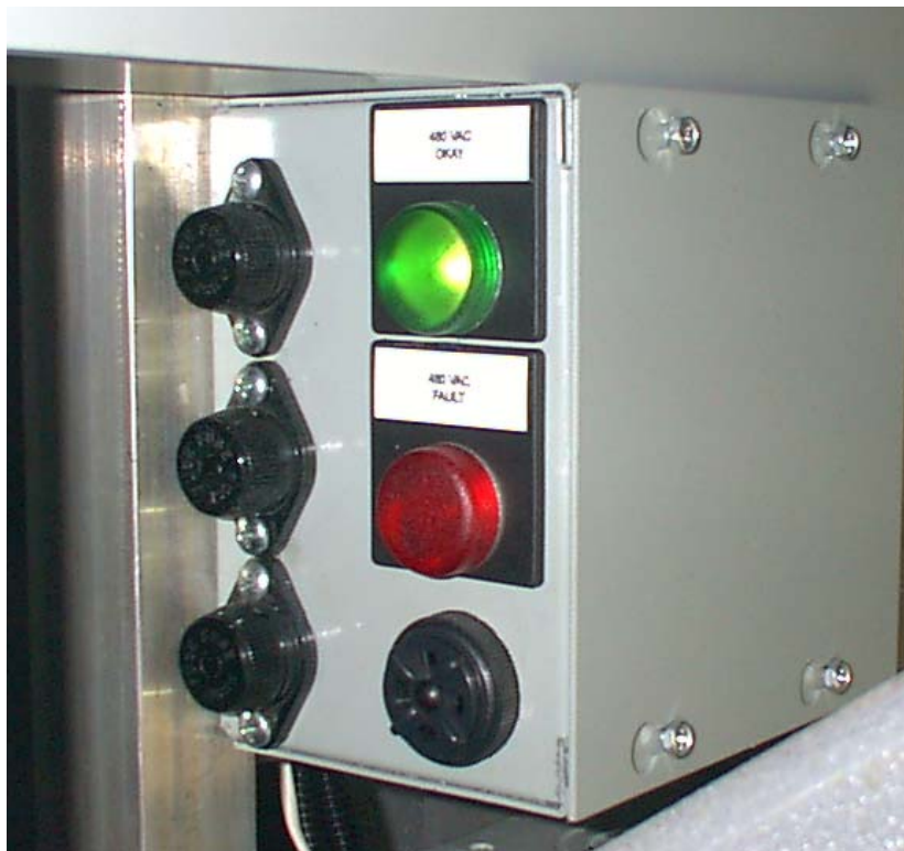
Figure 29: 480V AC Phase Power Monitor
