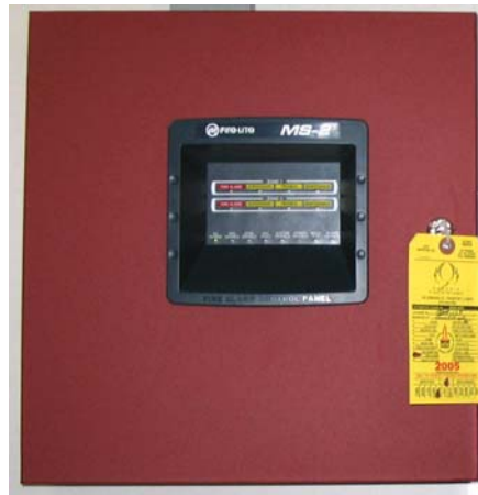
Figure 19: Fire Alarm Control Panel
