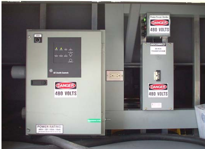
Figure 25: Automatic Transfer Switch and Phase Power Monitor
