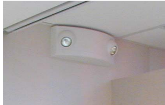
Gantry Room Emergency Light
