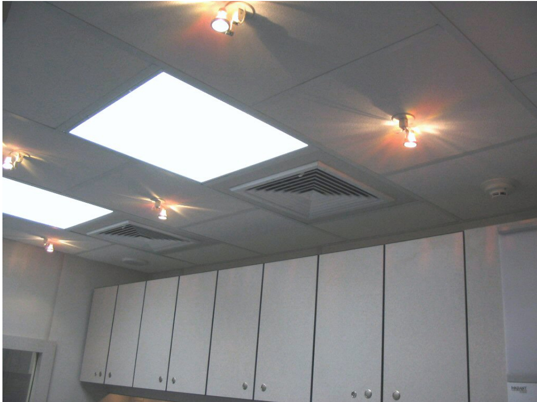
Figure 46: Control Room Overall Lighting
