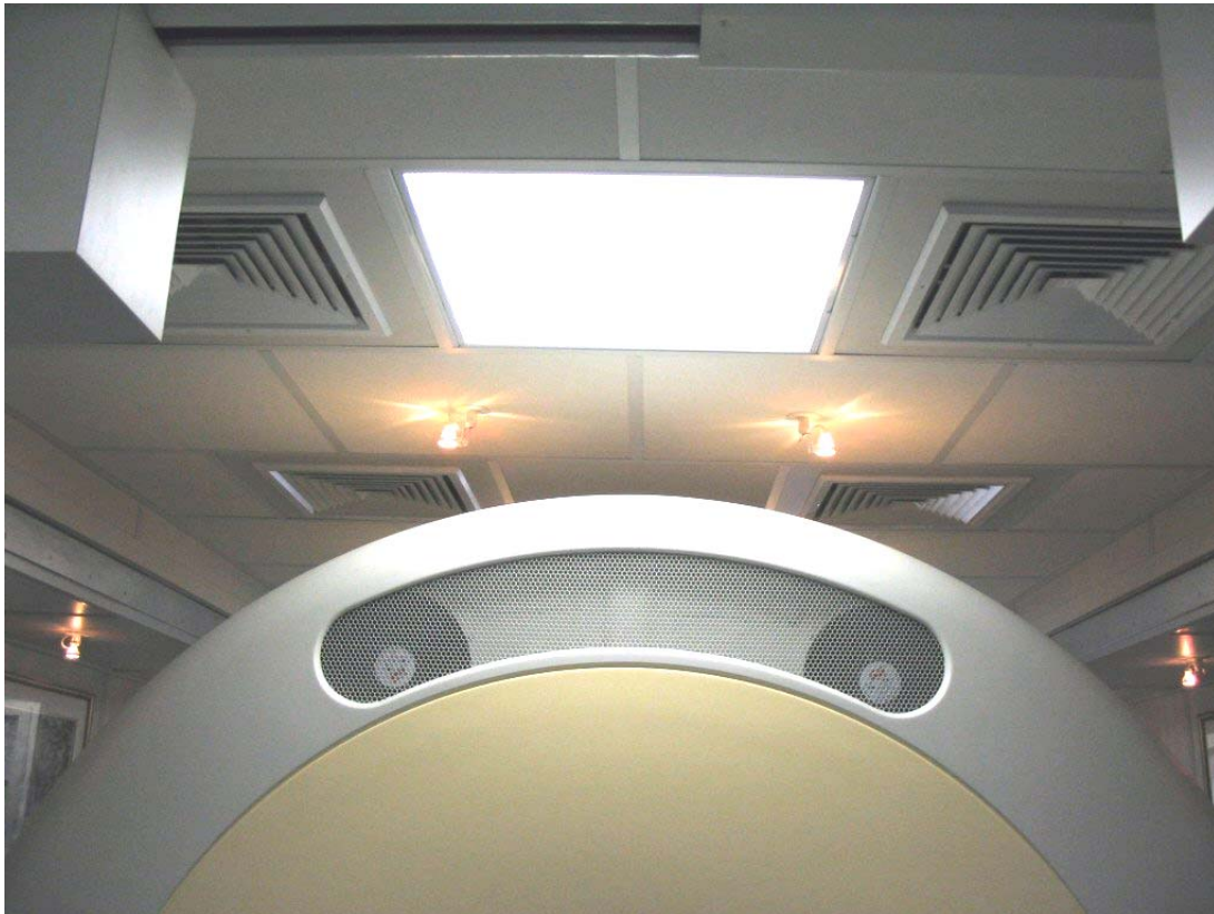
Figure 47: Gantry Room Overall Lighting
