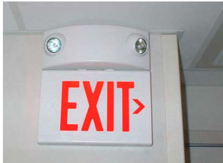
Control Room Emergency Light
