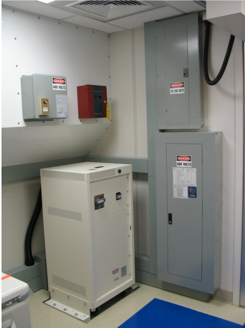
Figure 27: 480V and 120/208V AC Electrical Panels
