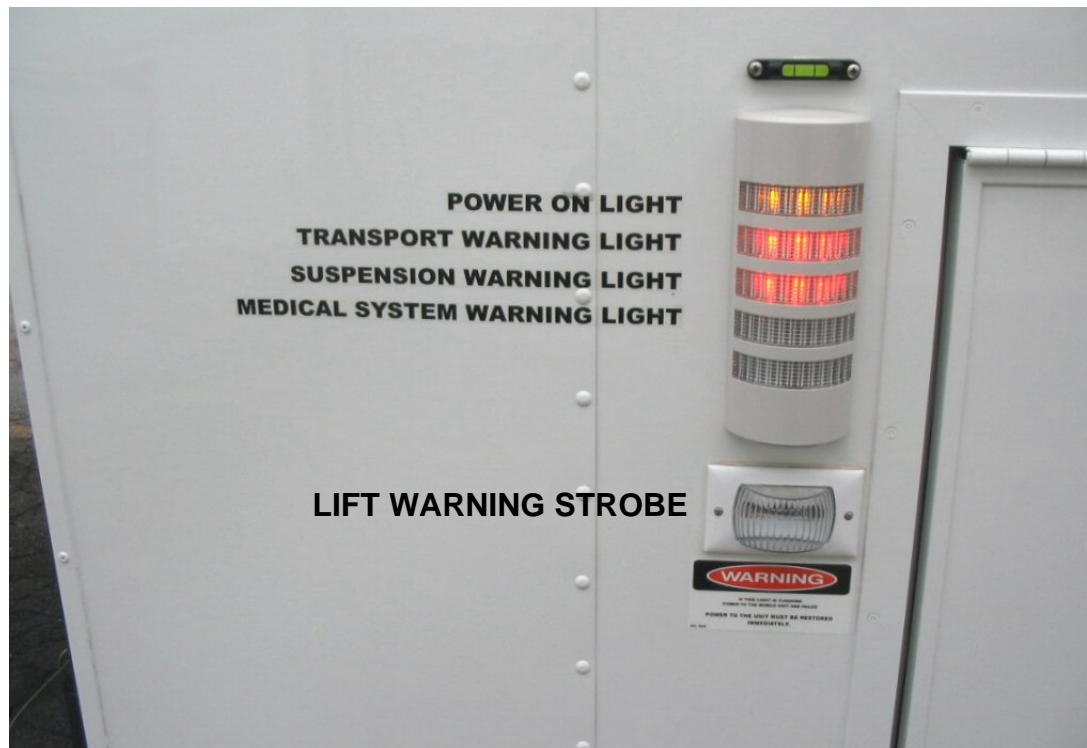
Figure 50: Lift Transport Warning Strobe
